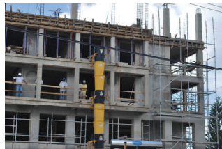
Chute being used to remove debris from upper floors to the ground.
