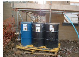
Recyclable waste placed in drums and ready to be removed from the site.
