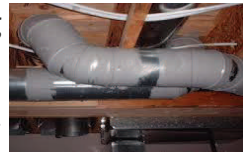
A resealed return duct.
