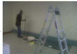
Painting without proper ventilation.
