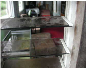
Dust on glass louvers
