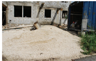
Wind action on this pile of grit can cause air pollution.
