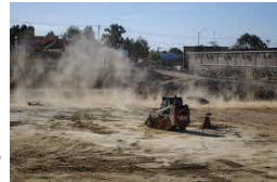
Dust being ejected into the air due to construction.
