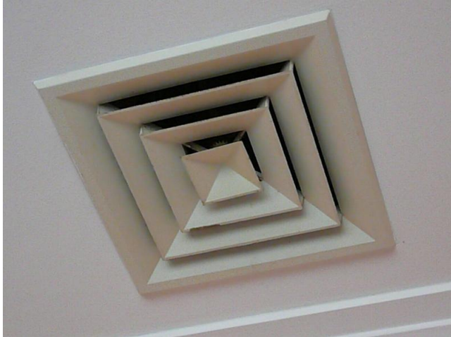
Figure 4: Typical diffuser vent
