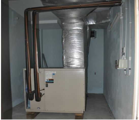
Figure 1: Evaporative component of the air handling unit, commonly referred to as the 'air handler'. This is usually located within an air-handling room.
