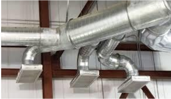
Figure 3: Ducts in ceiling
